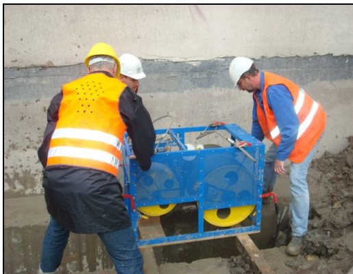
Picture 2: Ultrasonic unit installed at the panel
